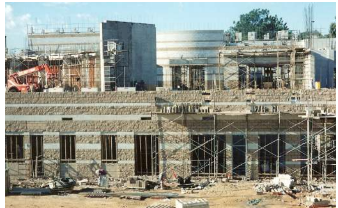
Construction began in March 2000 on Beth Israel's third home, a campus reminiscent of the Old City of Jerusalem.
